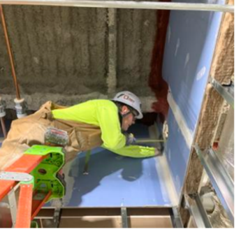
Paradise Fire Penetrations
